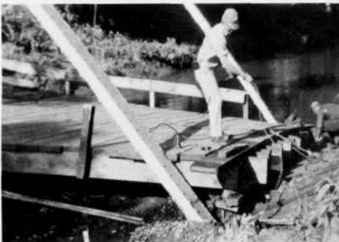
Demolishing old bridge on County Road 4 on border of Eldorado and Caledonia Townships.
